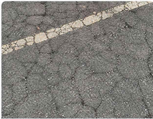
Parking lot — NE corner — Alligator cracking crack-filled.
