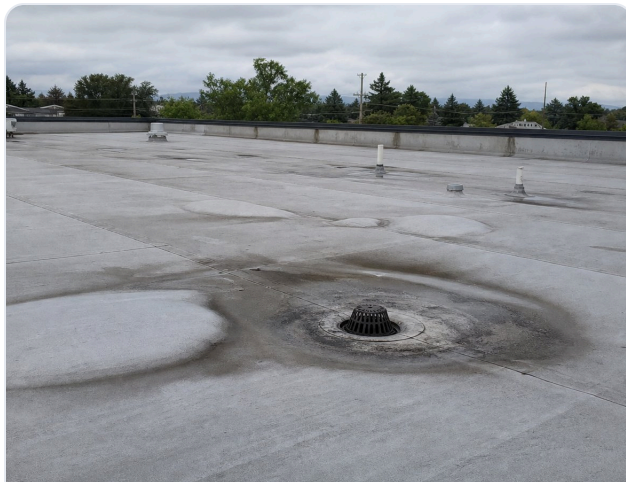
Roof membrane — north bay — Blistering and ponding near the primary drain; seams resealed.
